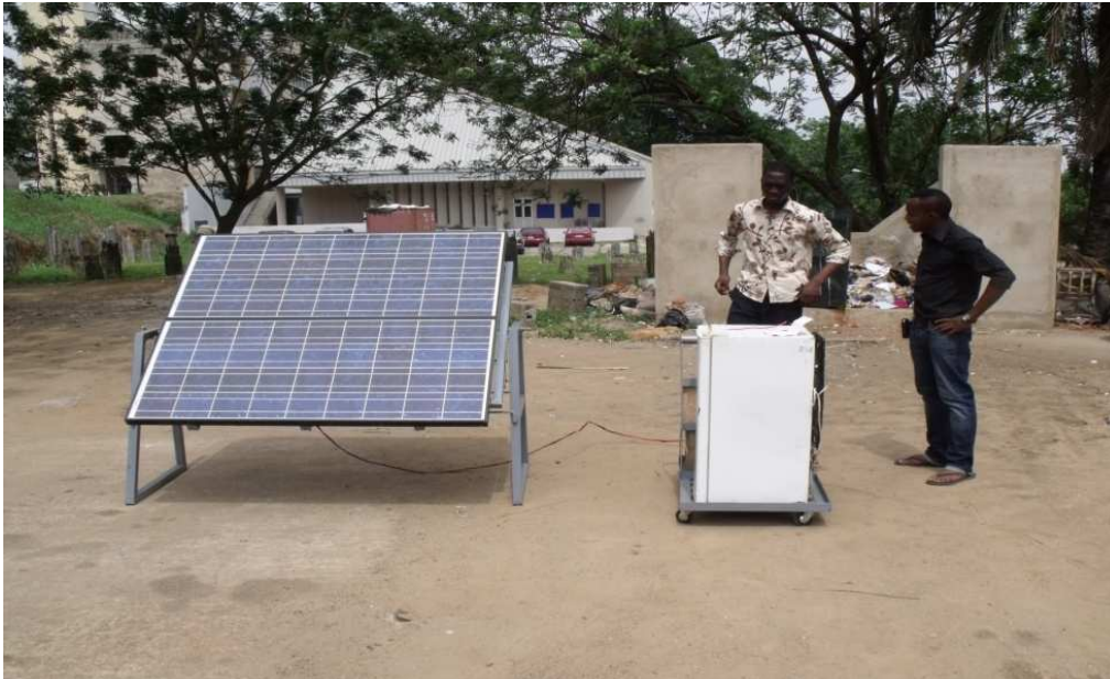
Figure 4: The Photovoltaic-Powered Vapour compression Refrigerator for Experimental Investigation.
